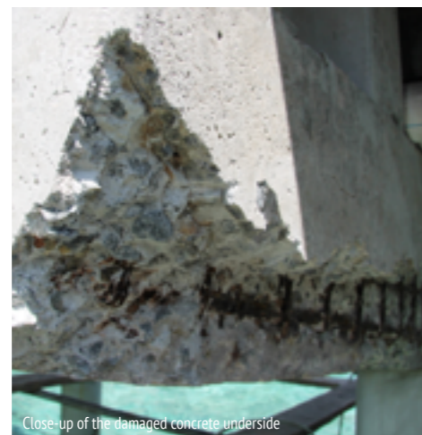
Close-up of the damaged concrete underside
