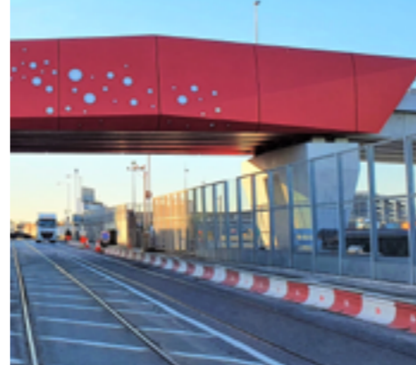
The Alexandra Road Bridge in Dublin was protected and embellished with MC-Color Flex.
